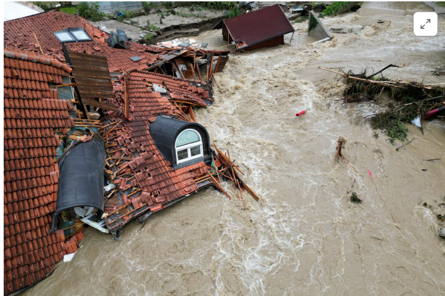
[5/5] A view of a damaged building in a flooded area, following heavy rains, in Prevalje, Slovenia August 6, 2023. REUTERS/Fedja Grulovic/File photo Purchase Licensing Rights
